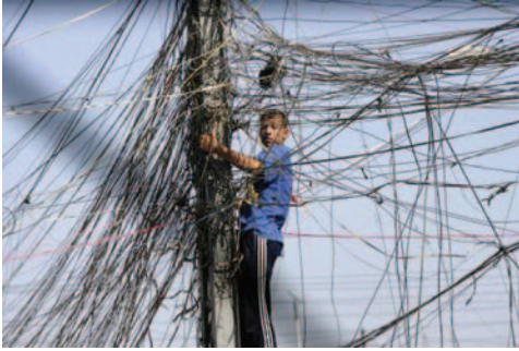
Figure 8. The shape of the electricity grid in Iraq – the linesman's view.
